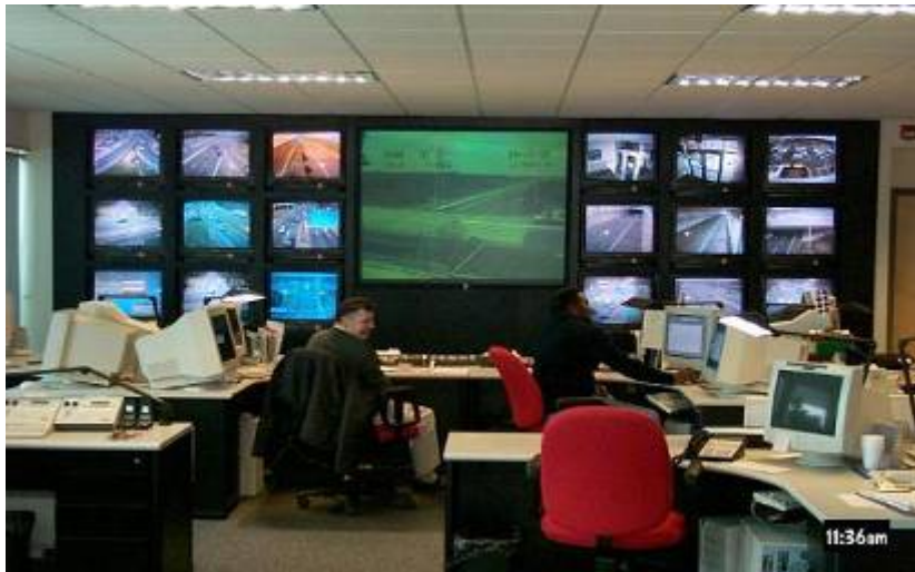
Traffic Operations Center-South
